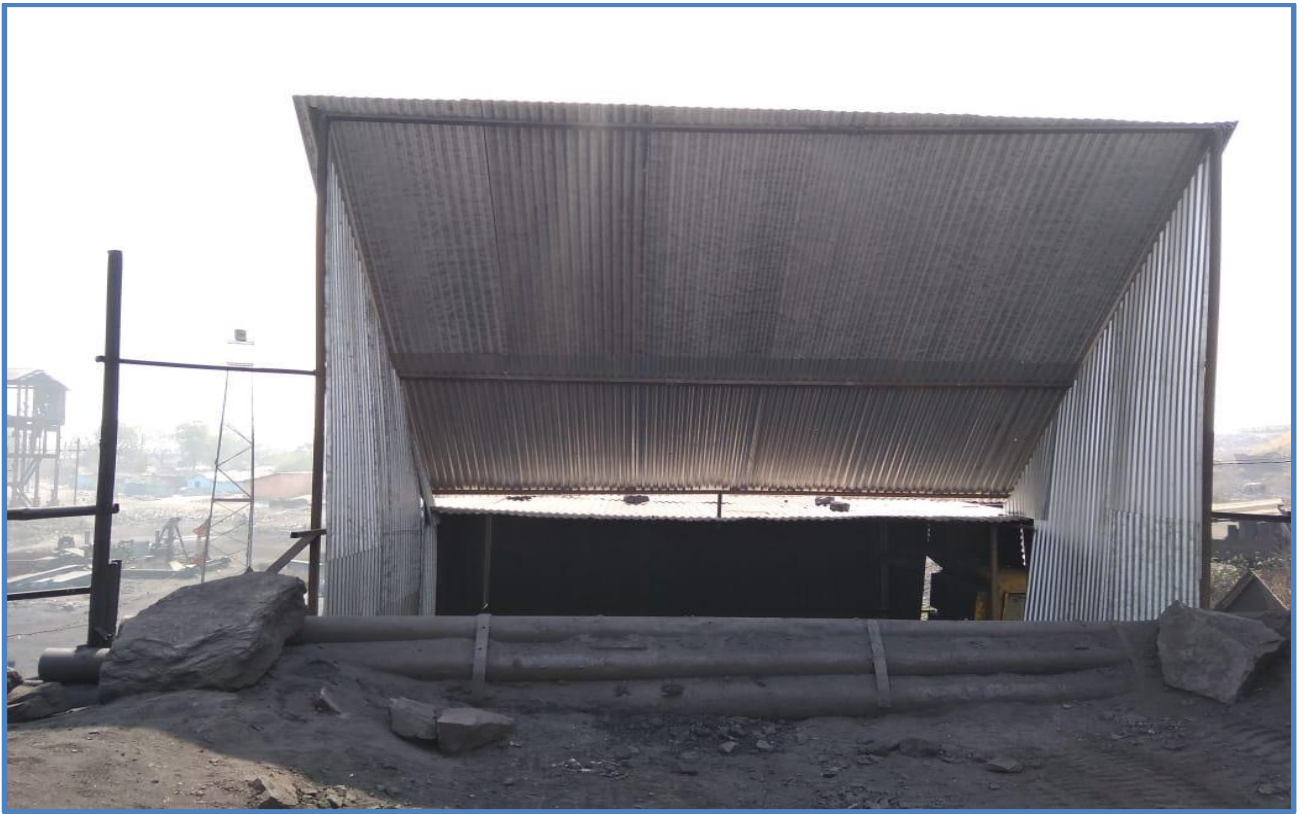
Picture 7 – Enclosed Coal Handling Plant
