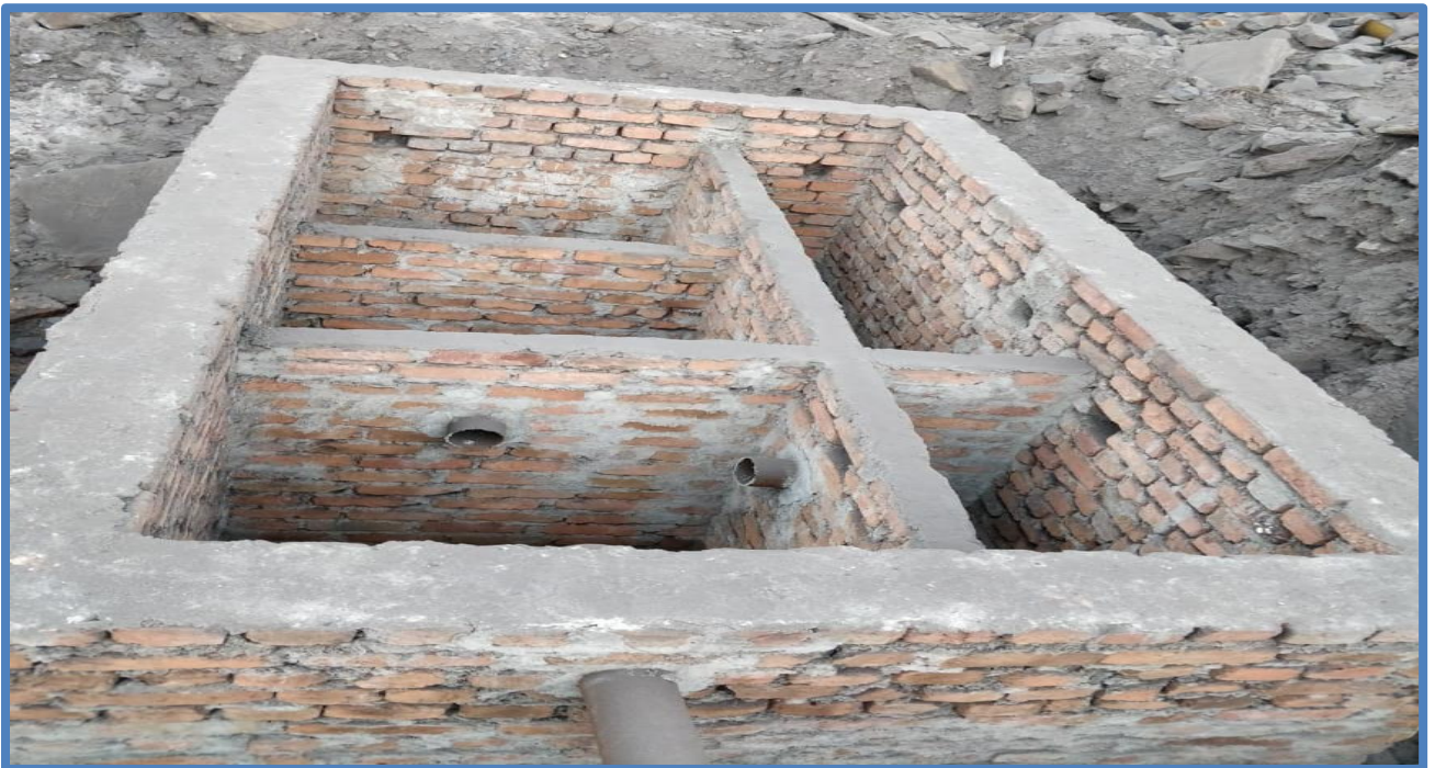
Picture 10 – Oil & Grease Trap
